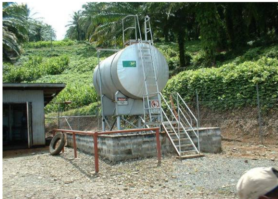
Plate 5: Bunding of bulk tank to AS 1940 – pollution prevention
